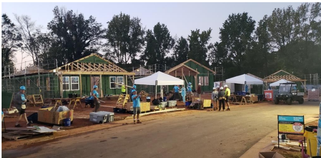
Figure 1. View at dawn of cul-de-sac on Jimmy and Rosalyn Carter Project build for Meadows at Plato Price community, October 2023, Charlotte, North Carolina. Photo by author.
